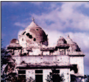
Damaged dome with holes made by shelling
